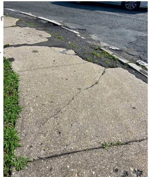
Figure 13: Image of curb ramp in West Springfield in disrepair and without accessible features.
